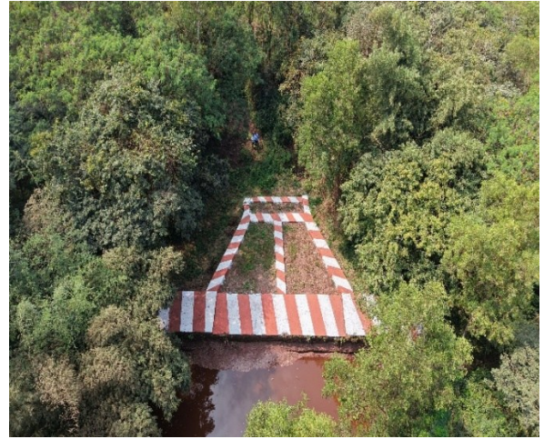
Check Dam outside Mining lease area
