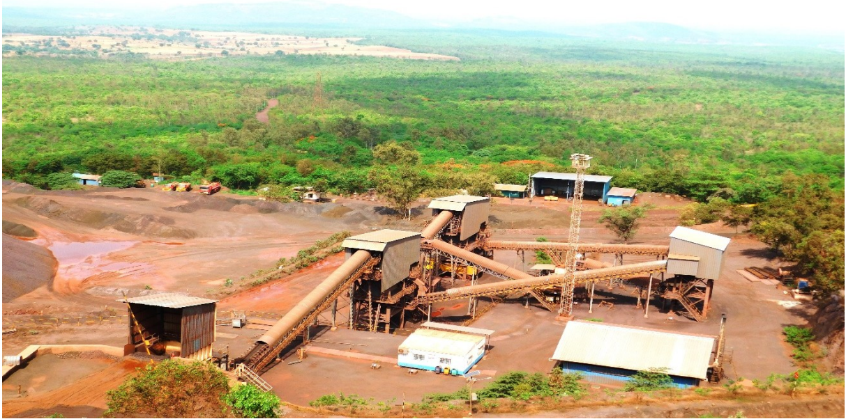
G.I. sheet hood cover on the conveyors of processing plant within the green ambient
