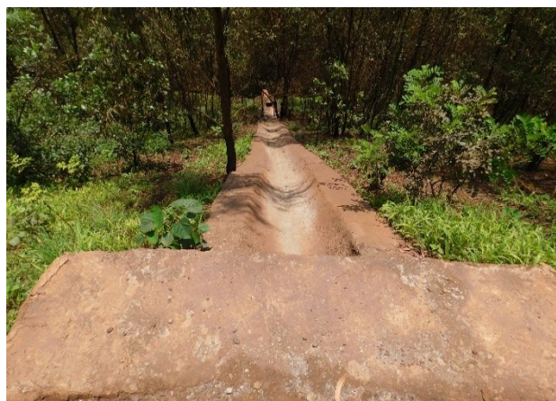
Vertical Drain on waste dump
